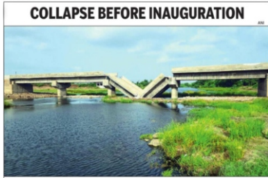
A bridge over the Mindhola river connecting Majpur and Degama villages of Gujarat's Tapi collapsed before its inauguration on Wednesday. No casualties have been reported from the site
